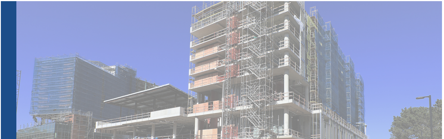
ADVANCEMENT™ LT was used in the construction of the UCSD North Torrey Pines Living and Learning Neighborhood.
